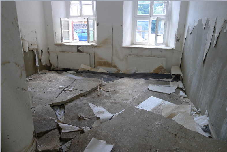
Schäden am Zementestrich (Goltz 2012)
