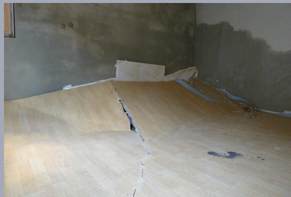
Schäden am Zementestrich (Goltz 2012)
